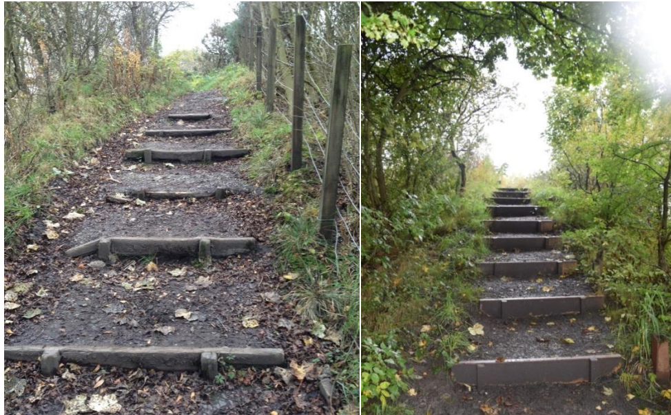
Bing on south shore – steps needing repair (left) and steps that have had repair by Paths for All and Education Community Learning and Development project (right).
