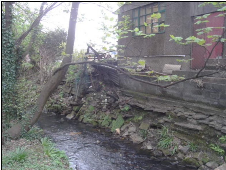
Failing Retaining structure adjacent to the Brothie Burn, Alloa - 15/04/09
