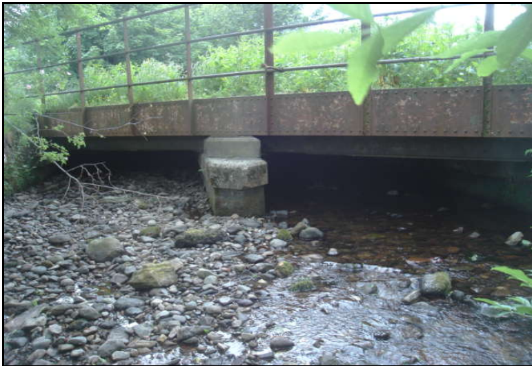
Build up of sediment beneath Mixed Leisure Route (Former Railway Bridge), Dollar Burn, Dollar - 22/06/09
