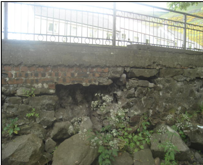
Damage to Retaining wall, Alva Burn, Alva - 28/05/09
