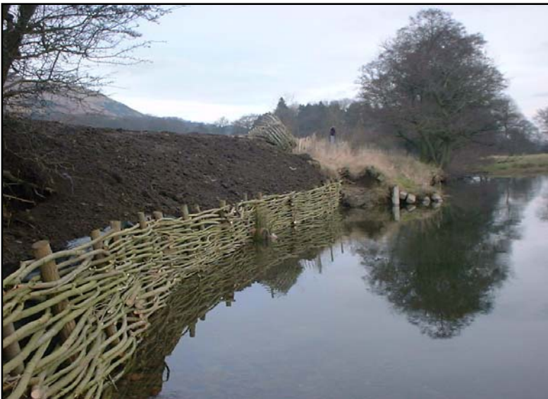
Willow walling of the north bank of the River Devon between Tillicoultry and Dollar
