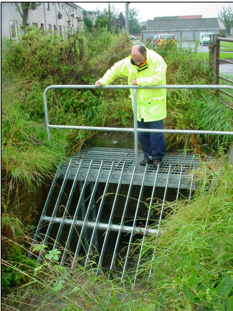
Photo 12 - New Trash Screen at Sauchie Burn Culvert - 10/08/04
