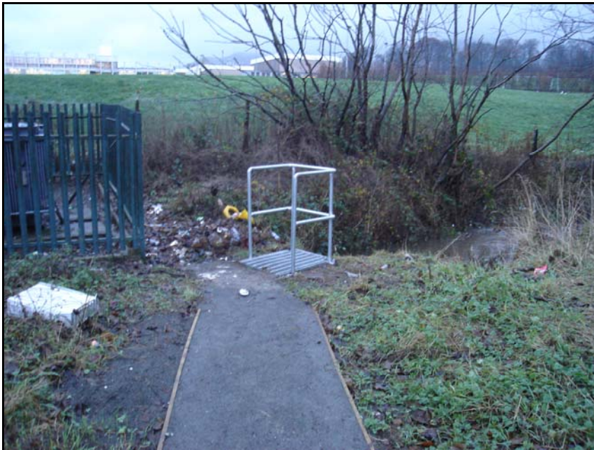
Photo 5 - Trash Screen, handrail and access installed at culvert entry north of Ormiston Drive, Alloa - 12/12/06
