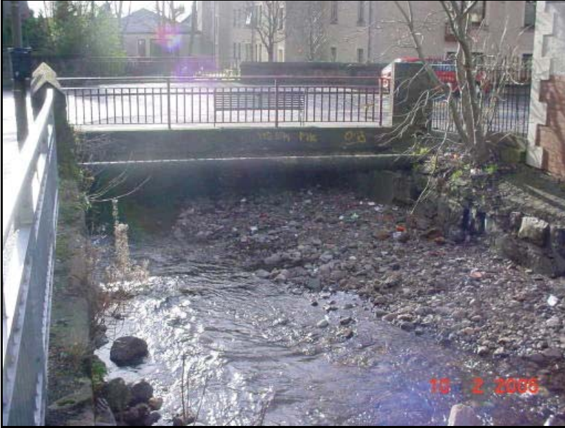
Photo 20 – Excessive build up of Sediments upstream of and beneath the A91 Road Bridge, Alva Burn Alva. – 02/10/05
