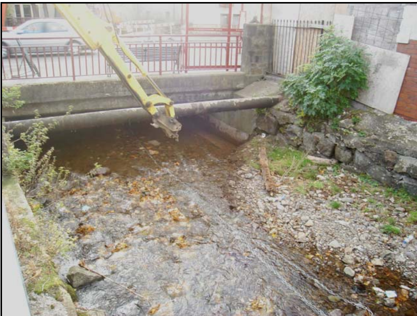
Photo 21 – “CAR” consented works to remove sediment from A91 Road Bridge, Alva Burn, Alva – 09/11/07
