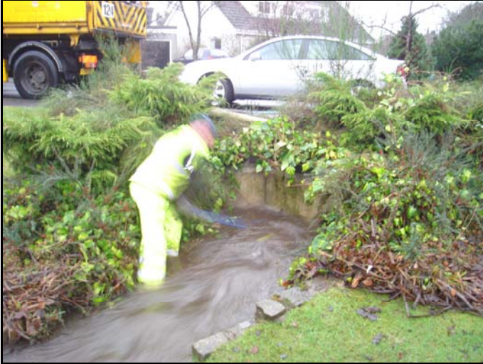
Photo 17 – Flooding issue being resolved by Council staff at Kirkhill, Muckhart – 12/01/07
